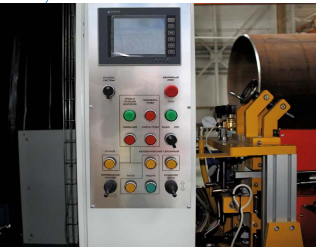
Front panel of control station
